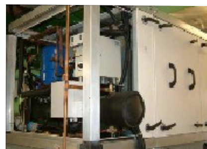
AHU Mounted Design
